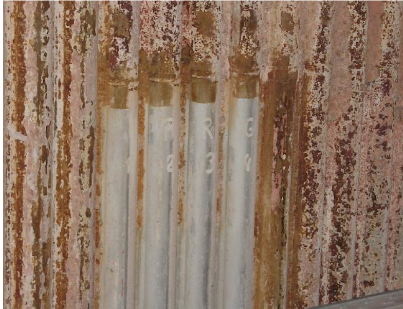
Fragment of a power plant boiler screen partially covered with a protective coating after a certain exploitation time
